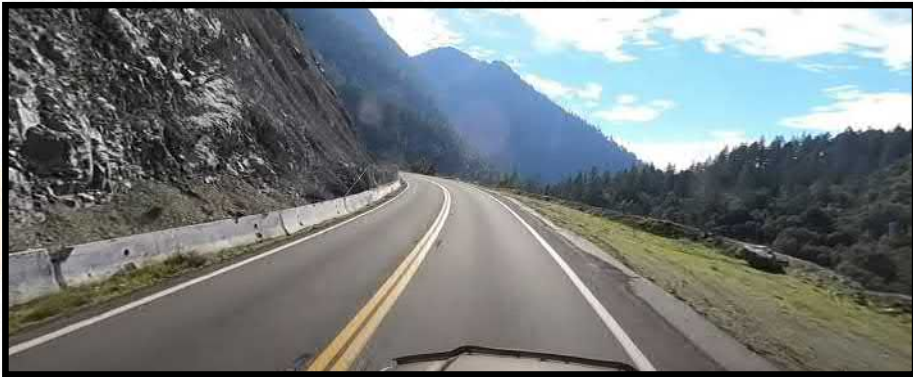
Rt 0096 - SR-96 Concern Area - drop off to river on Right
