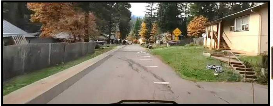
Rt 0110 - Shan D Dr. water coming up through pavement
