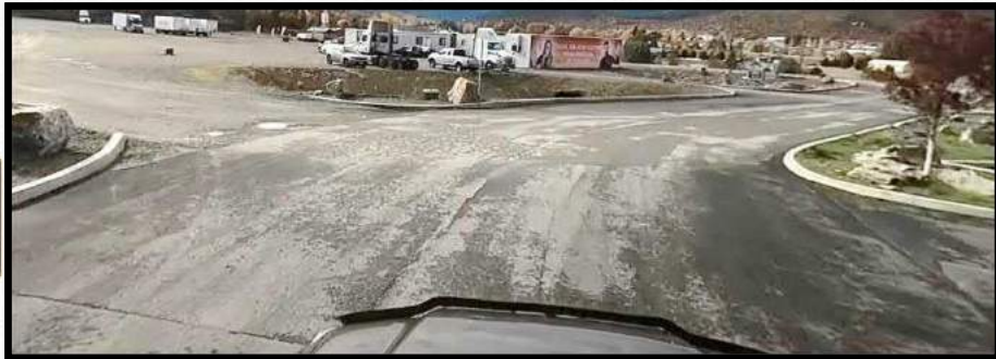
Rt T054_030(2) - Casino Way Entrance to Overflow Parking Alligatored
