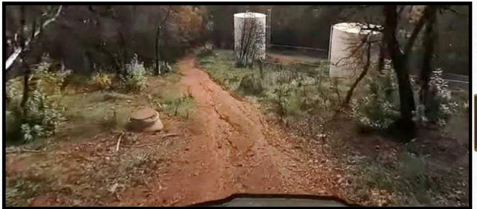
Rt 0111_015(3) - Itroop Rd Erosion
