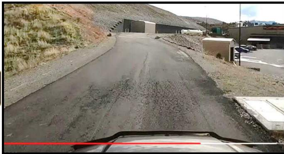
Rt T054_020(2) - Casino Way Alligatored Area
